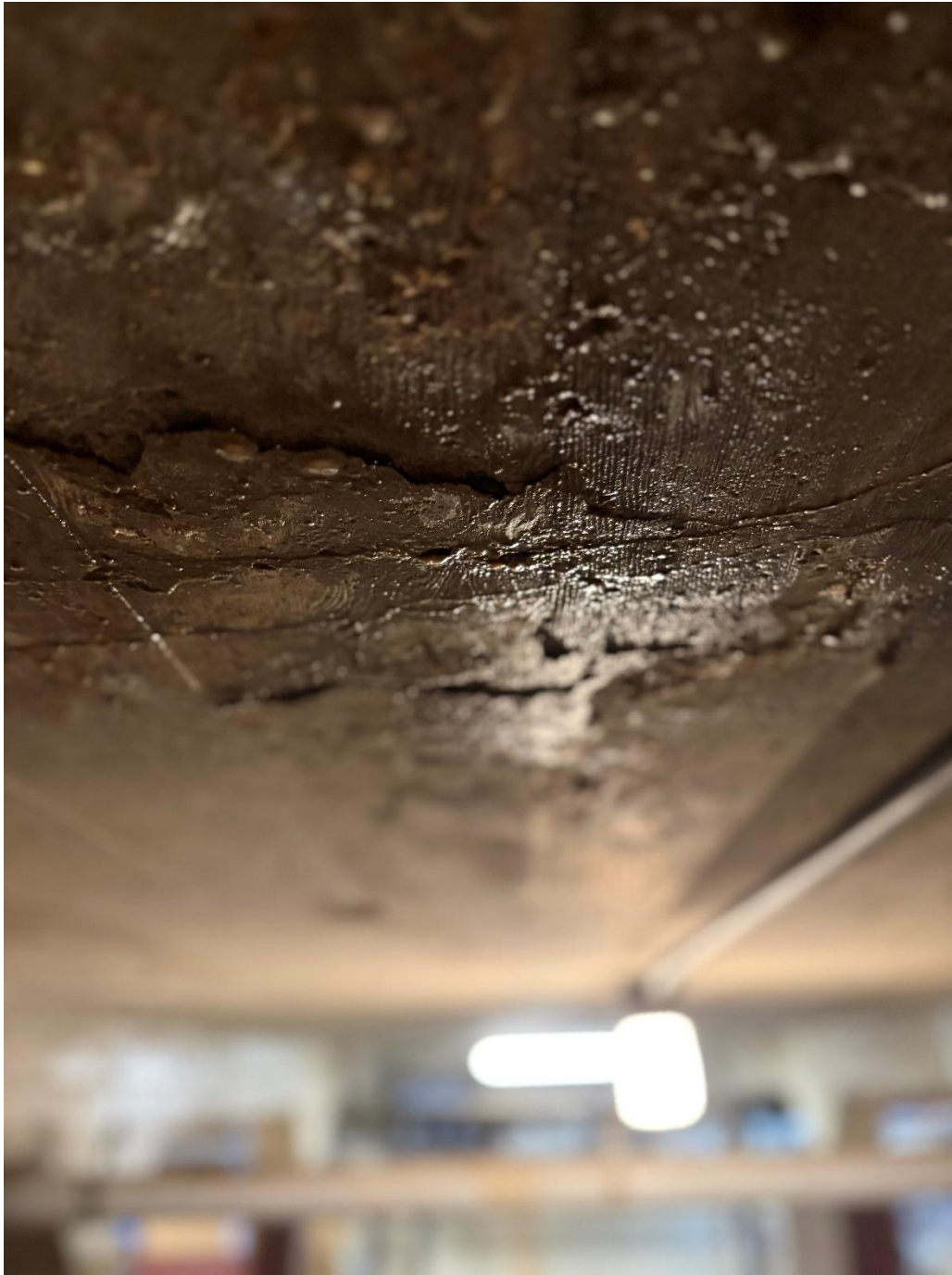
Photo 4 – Concrete spalling along line 3.2
