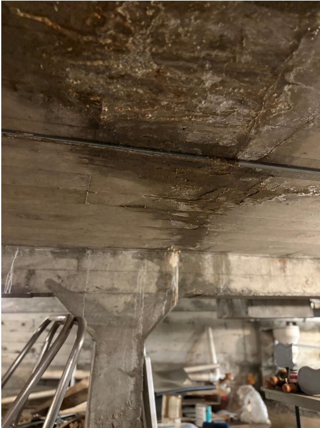
Photo 3 – Cracking in concrete pool shell with water intrusion
