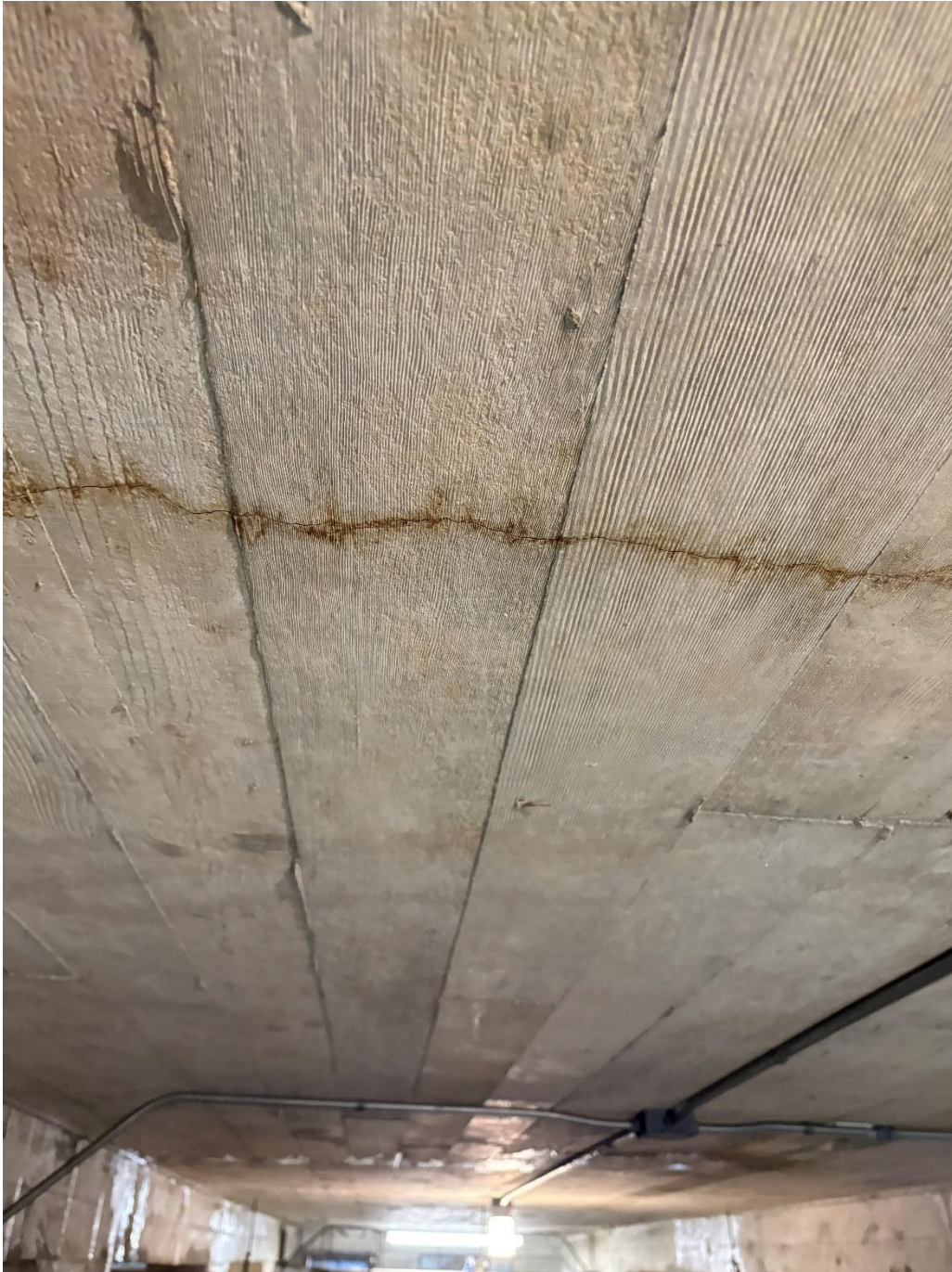
Photo 1 – Transverse cracking in concrete pool shell
